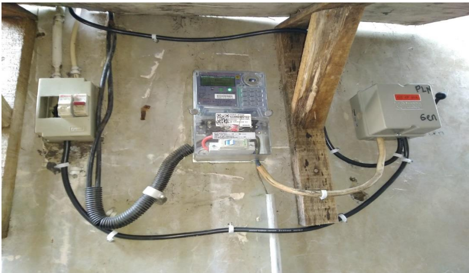
Gb. 1. KWH meter serta handel PLN/Genset
